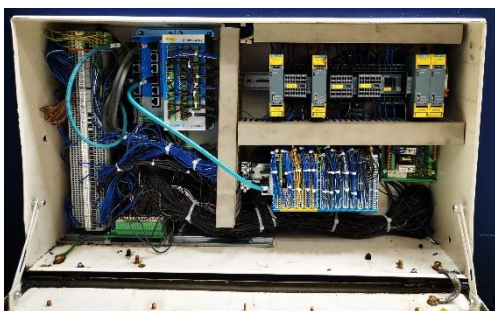
Closing control, completely converted to current MC6 modules
