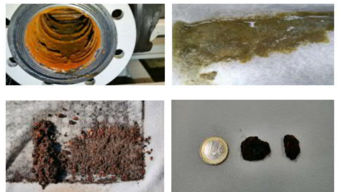
Examples of deposits: Biology, corrosion and lime
